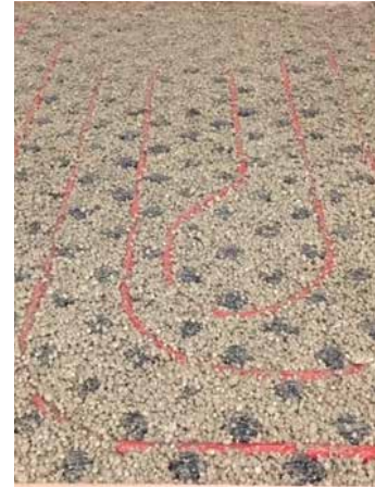
3. Flat deduction of SYMPOR-LB 400 (or Sympor LB 400 S) directly at the top edge of the nubs
