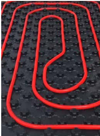
1. Installation of Sympor Unisolo 14-17 on a clean surface. Insertion of floor heating pipes
